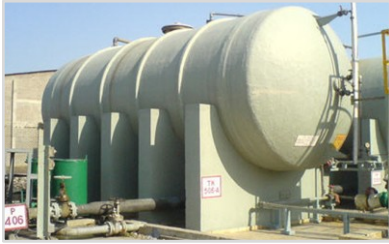
Water & Chemical Storage Tanks
