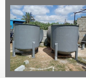
Continuous Leachate Treatment Tanks
