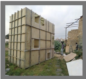
Rectangular Effluent Treatment(ETP) Plants
